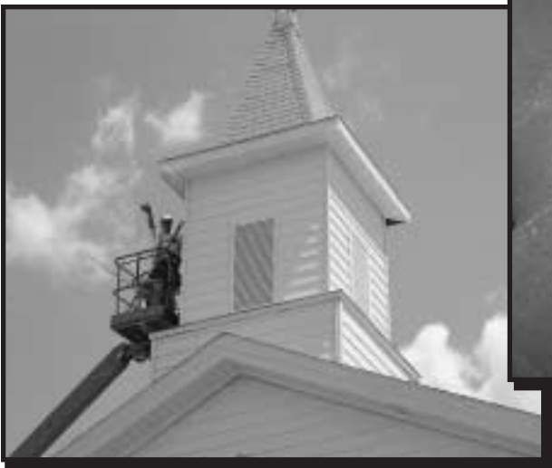
Greg and Chad are putting the final touches on the steeple (above) and the bell's clapper (right) needed some repairs before it would ever ring again. The tape measure shows that this clapper is over four-feet long.
