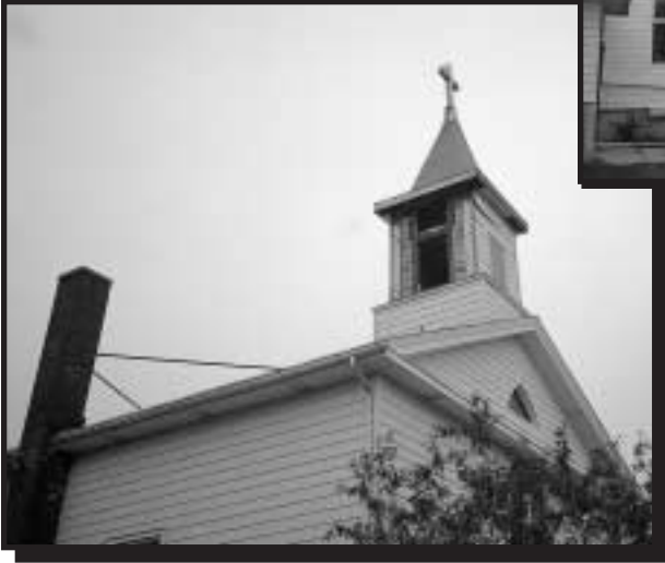
The exterior of the Darien Community Baptist Church's steeple (above) was ready for repair, and with the assistance of a 65-foot boom truck, Greg Mueller and Chad Maass were able to start the project, safely.
